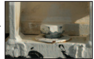
This bolt is loose and the joint is generally lubricated.
