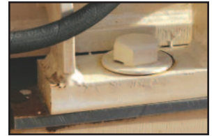
This side restainer bolt is too tight.
